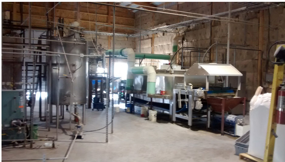
A look inside the Montana Microbial Products pilot plant in Melrose, Montana. Photo courtesy of MMP.
