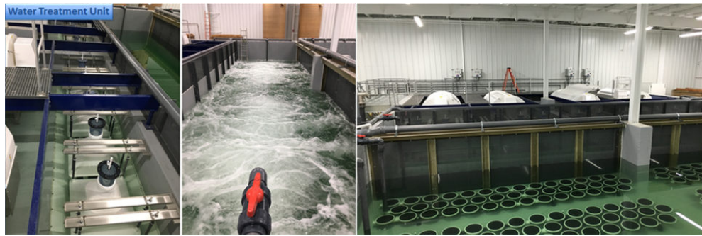
Views of the water treatment unit.
